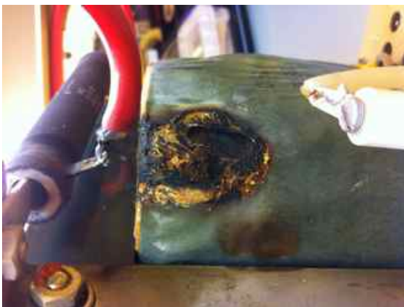
Transformer case charring
