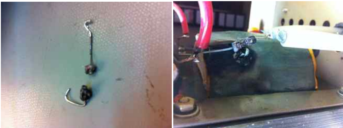
Failed resistor and transformer damage
